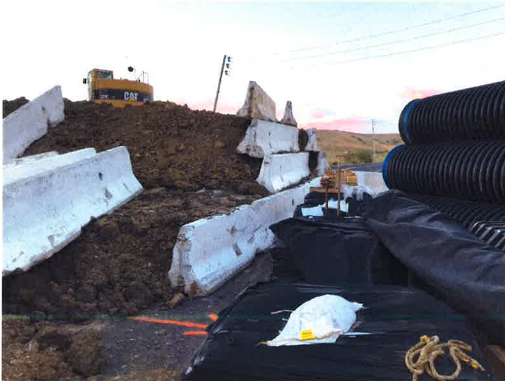
Soil being stockpiled at Pinole Valley, Castro Ranch and Alhambra Valley roads.
